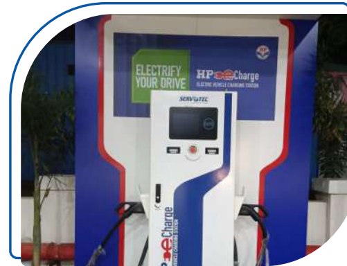
Glimpse of HPCL Project
